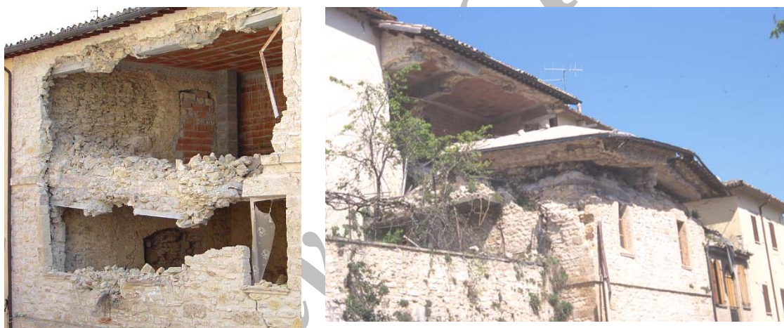
Figure 1. Example of a) Out-of-plane collapse of a wall with r.c. tie beams, b) roof hammering the masonry walls
