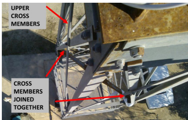
Fig. 10 Photo (taken from above the tower) showing the upper cross members joined together by a single bolt
