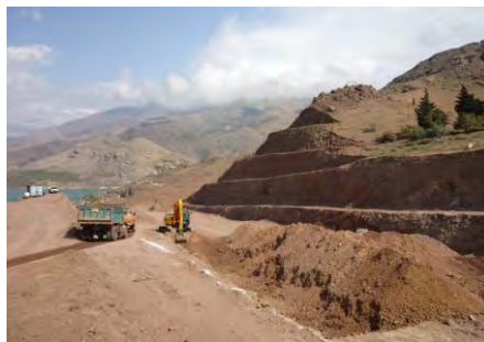
Figure 2. A view of the cutting slope with four berms of 4 m width and 6 m height (1H: 2V) and heavy works during the 5-6 m excavation on the toe of slope along 41+400 to 42+200 km of Qazvin-Rasht freeway
