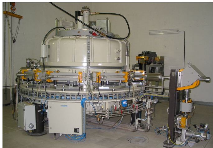
Figure 2. Rhodotron accelerator model TT-200 (IBA Co., Belgium) installed at the Yazd Irradiation Center, Radiation Applications Research School, Atomic Energy Organization, Iran.
