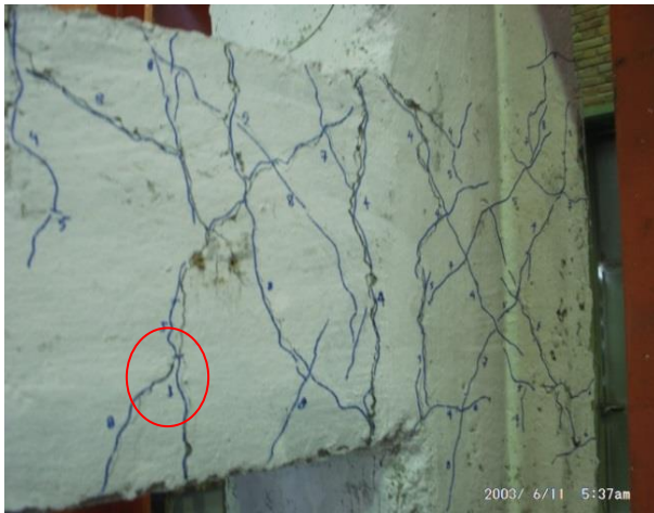
Fig.5-Location of first crack
