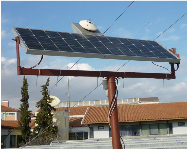
Fig. 1 PV panel, motorized mount and pyranometer configuration on the rooftop of the lab
