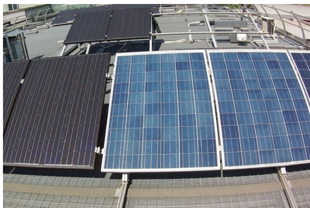
Fig. 7 Visual analysis of PV modules in Solar Tech Lab
