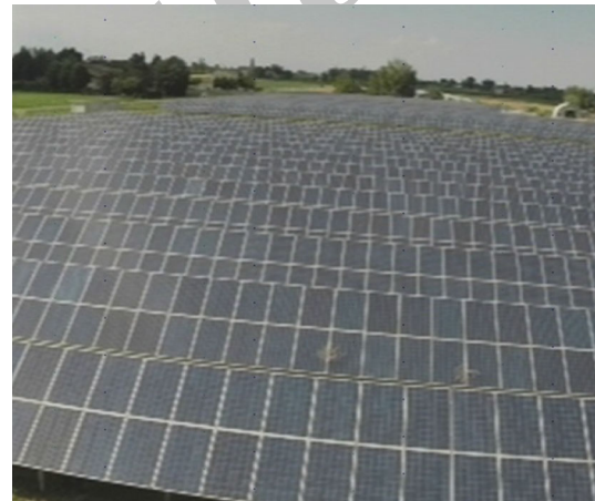
Fig. 3 PV plant in North of Italy
