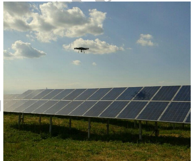
Fig. 6 PV modules inspection at PV plant in north of Italy by Nimbus PPL-610 UAV
