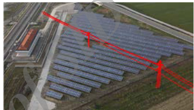
Fig. 12 PV plant crossed by a MV line under analysis
