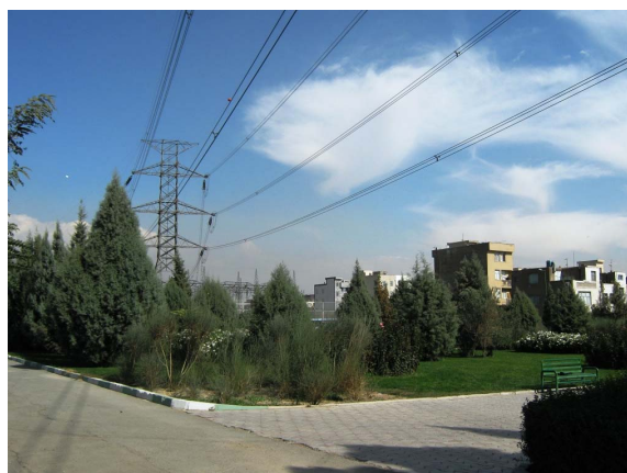
Fig. 1: 230kV overhead transmission line near a public park, Azadegan Substation
