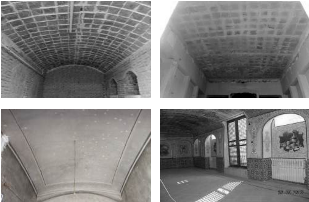
Fig. 16. A few Qomi-poosh vault samples with different deflection (Source: architect Helli's personal archive).
