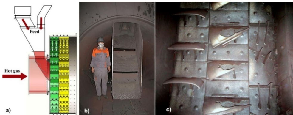
Figure 1. a) Schematic view of dryer and feed chute, b) feed chute, and c) worn dryer flights.
