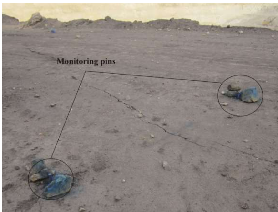
Figure 5. The installed monitoring pins to monitor the displacements around the F-a fault hanging wall on top of the slope under study. Tension cracks are observed around these pins.
