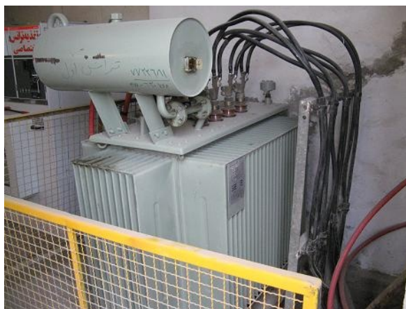
Figure 4. The picture of 400 kVA distribution transformer
