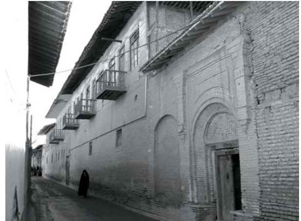
Fig. 5: Main façade of the house from the northern passage before the restoration operation
