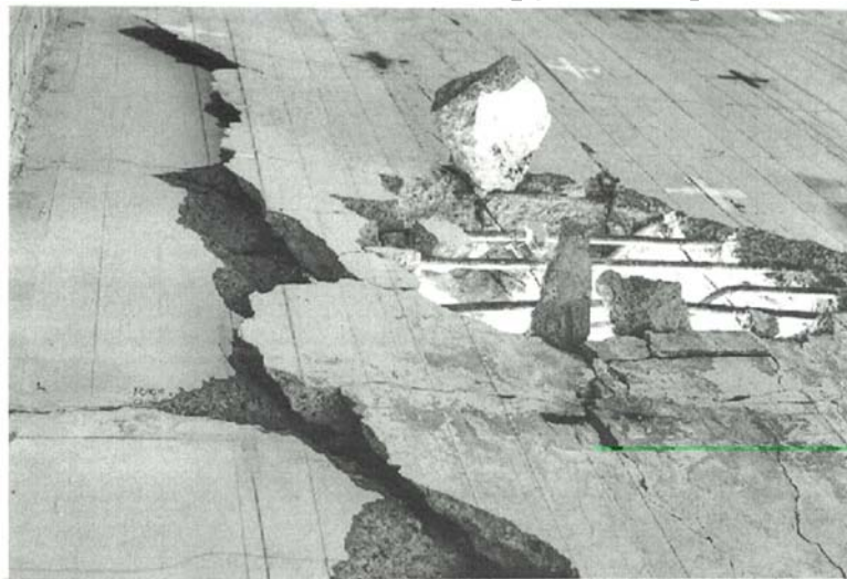
Figure 2 A typical punching shear failure of a bridge deck
