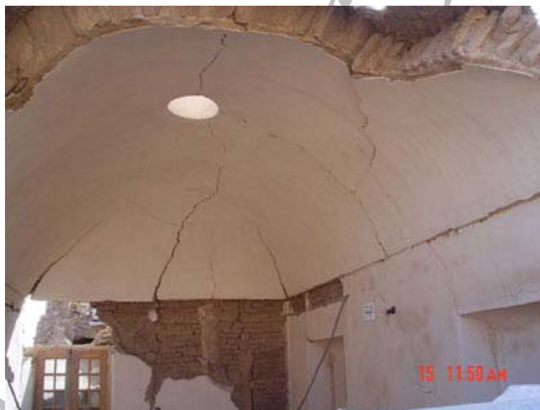
Figure 7. A vault with cracks in Arg-e-Bam
