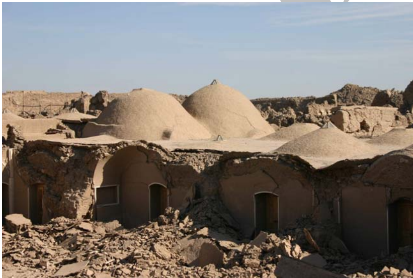
Figure 11. A meridian cracks in the dome
