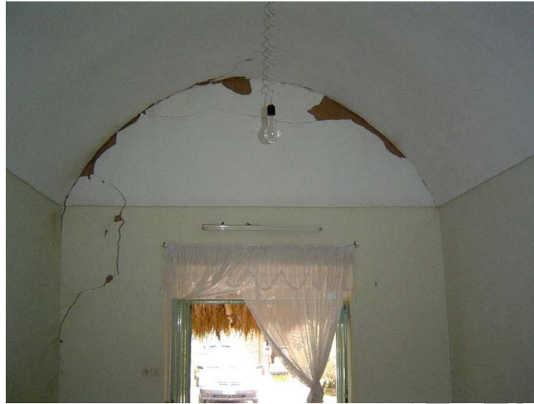
Figure 6. Cracks at the intersection line of the vault with the end plate
