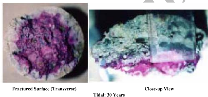
Figure 4. Appearance of the fractured surface after spraying phenolphthalein solution
