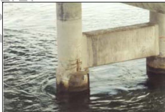
Figure 19. Bridge on the Florida Keys. Critical corrosion of epoxy coated reinforcement
