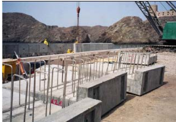
Figure 17. Stainless steel reinforcement used in the precast structural members to replace a corrosion damaged seawall protecting the existing important buildings and the new Building Complex (Figure 15) from the Gulf.
