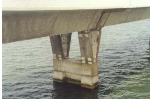
Figure 20. Bridge on the Florida Keys. Critical corrosion of epoxy coated reinforcement leading to splitting of the V formed supports now strengthened by prestressed bolts
