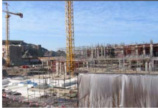
Figure 15. Overview of the construction site of a seaside Building Complex. Stainless steel reinforcement is used in the outer exposed structures from below ground water level up to level +5m. See Figure 16.
