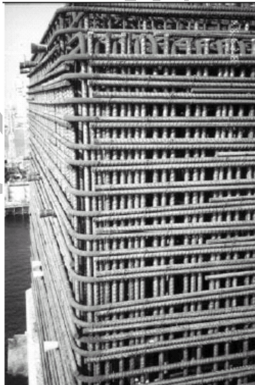
Figure 11. Example of reinforcement detailing which does not respect the need for reliable casting and compaction of concrete. Particularly the quality of the concrete "skin" (the cover) is in danger
