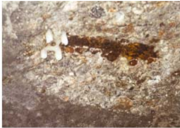
Figure 12. Plastic spacers allow direct access of chlorides to the reinforcement
