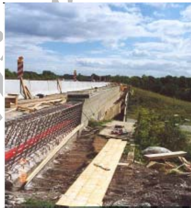
Figure 18. Replacing edge beams and parapets on Danish bridges and crash barriers on the motorways exposed to de-icing salt. SSR is introduced to avoid future repairs as well as avoiding the serious delays and inconveniences to the users, an issue becoming more and more in focus with the growing awareness of the costly societal consequences of such delays.
