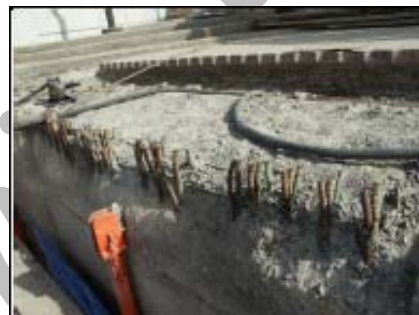
Figure 21. Seawall reinforced with epoxy coated reinforcement-heavily damaged by reinforcement corrosion after about 12 years
