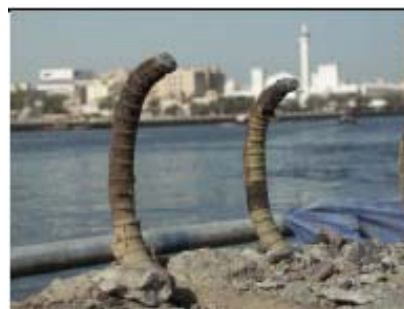
Figure 22. Close-up of the corroded epoxy coated reinforcement shown on Figure 21
