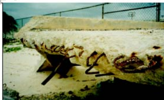
Figure 14. Close-up of the land based remaining parts of the “new” pier of which part of the remaining piles are shown in Figure 13. This pier was reinforced with ordinary black steel reinforcement and lasted only about 10 years.
