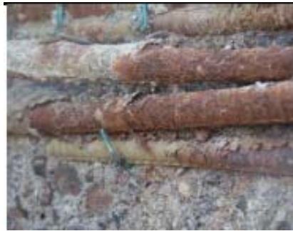
Figure 23. Details of the corroded epoxy coated reinforcement shown on Figure 21. The loose layer of epoxy on the corroding bar is clearly visible
