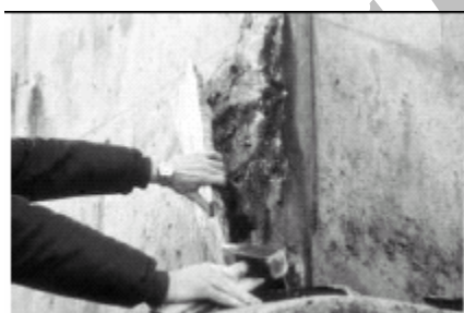
Figure 5. Bridge piers exposed to a temperate Nordic marine environment. Extensive damage in the splash zone after 18 years due to chloride induced reinforcement corrosion
