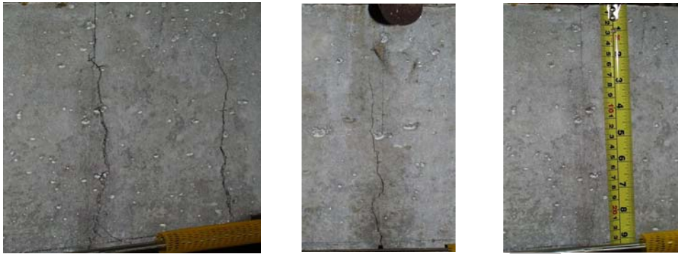
Figure 3. Measuring the crack width
