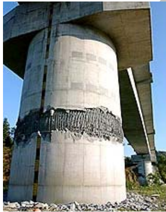
Figure 3. Severe but promptly repairable damage
