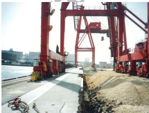
Figure 5. Heavy distortion of quay wall in
