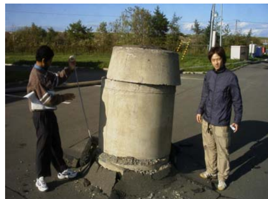
Figure 6. Significant floating of sewage
