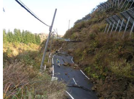
Figure 4. Fatal collapse of rural road after 2004 Chuetsu earthquake in Japan
