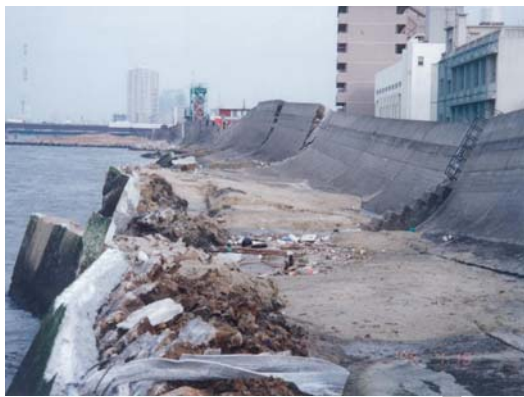
Figure 7. Significant subsidence of Yodo River dike in 1995 (Ministry of Construction)
