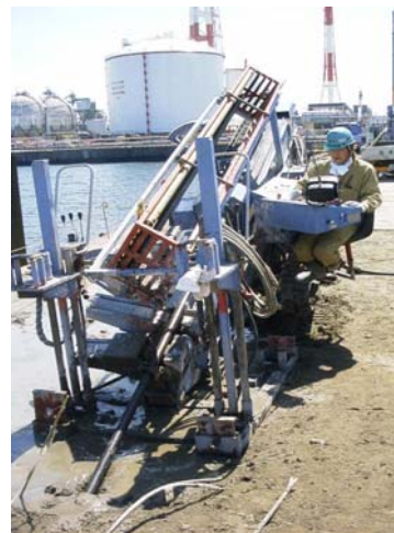
Figure 12. Soil improvement by means of silicate grout under existing structure in the vicinity of quay wall
