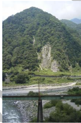
Figure 18. Slope reinforcement to prevent its failure and production of debris (mitigation at source)
