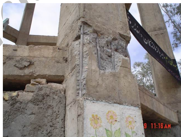
Figure 15. Clos-up view of the cracks in the structural joints of the elevated reinforced concrete water tank tower (note the rebars with no threads).
