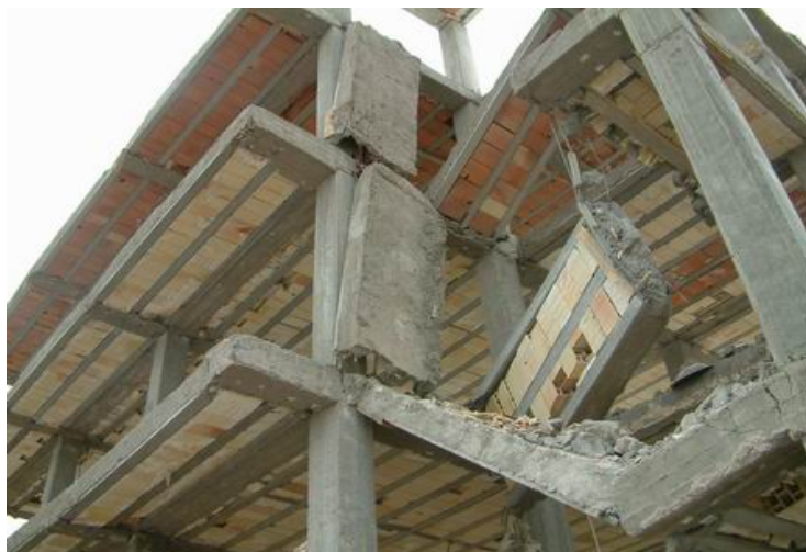
Figure 11. Poor performance of stairs in reinforced concrete structures
