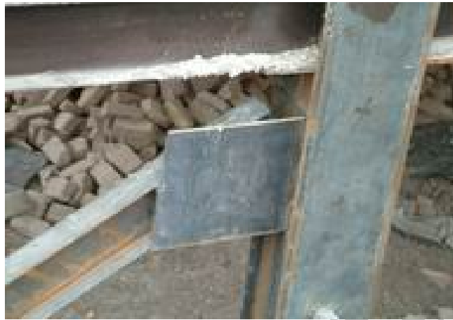
Figure 9. Incorrectly bracing with single I shaped brace only connected to the column
