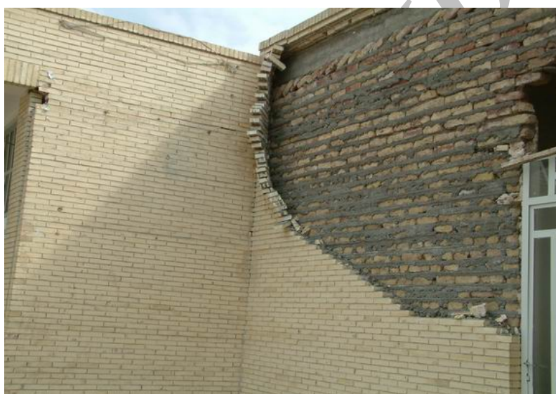
Figure 6. An example of reinforced brick buildings in the earthquake-affected area with a relatively good performance
