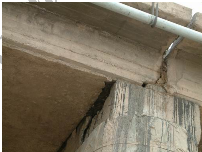
Figure 17. Separation of bridge Spans from the abutment
