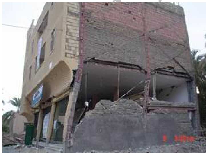
Figure 10. Unacceptable bracing system where the cross-section of bracing member is insufficient
