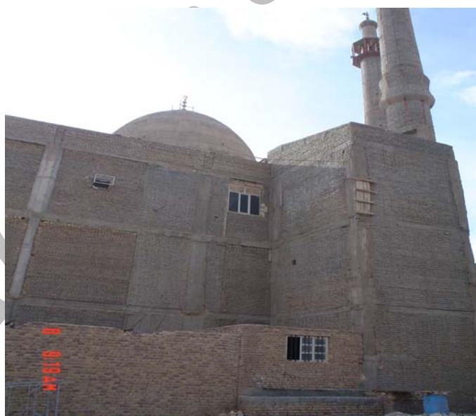
Figure 13. A reinforced concrete mosque after the earthquake which had a satisfactory performance
