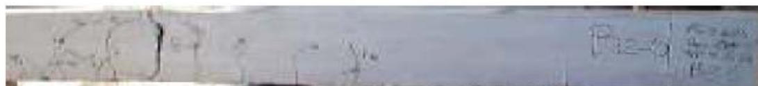
Figure 5. Typical flexural failure mode of the beam at longitudinal steel \rho \leq 1\% and no web reinforcement. ( \rho = 0.73\% , a/d = 5.5 , span=321cm)
