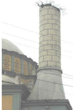
Figure 1. Damage to cylinder mid-height
