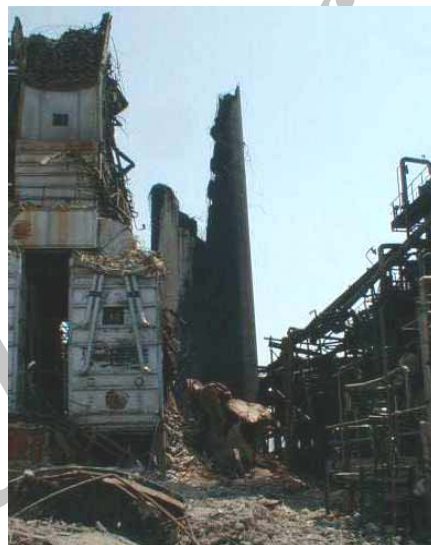
Figure 3. Remnants of failed stack
