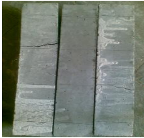
Plate 5. Cracking pattern of prisms
