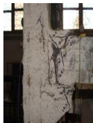
Figure 11. Failed cleat Angle connection
