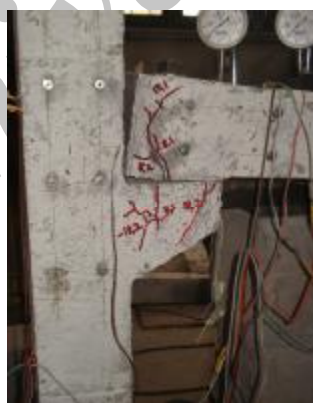
Figure 10. Failed J-bolt connection
