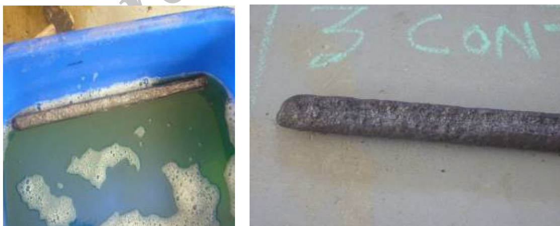
Figure 11. Typical view of cleaned rebar and view of reduced cross section
