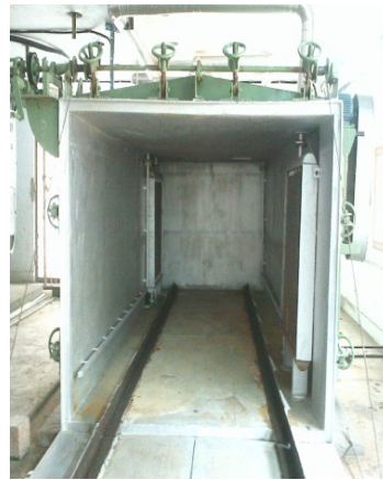
Figure 3. Steam curing chamber
