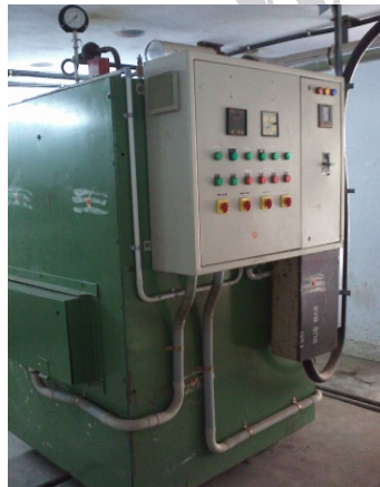
Figure 2. Steam boiler and controls
