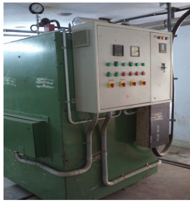
Figure 2. Steam boiler and controls
