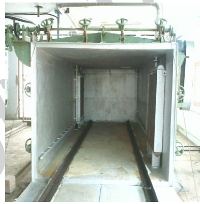
Figure 3. Steam curing chamber
