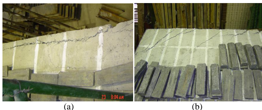
Figure 14. Cracked Shape of Concrete Slab of the Composite Diaphragms after Failure. (a) First specimen. (b) Second Specimen
