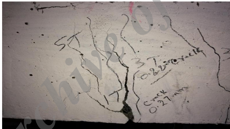
Figure 8. Crack width and Crack pattern of the 50 mm clear cover of M25 grade of concrete beam
