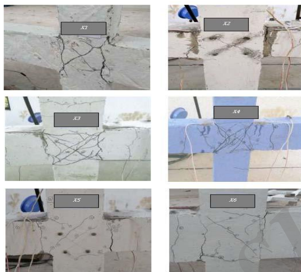
Figure 5. Damage patterns of test specimens
