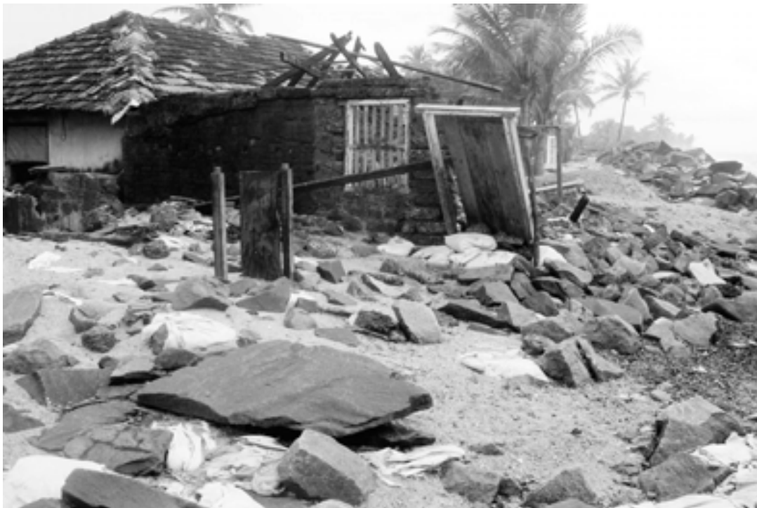
Plate 1. Loss of beach and property at Kotepura due to impact of storm waves
