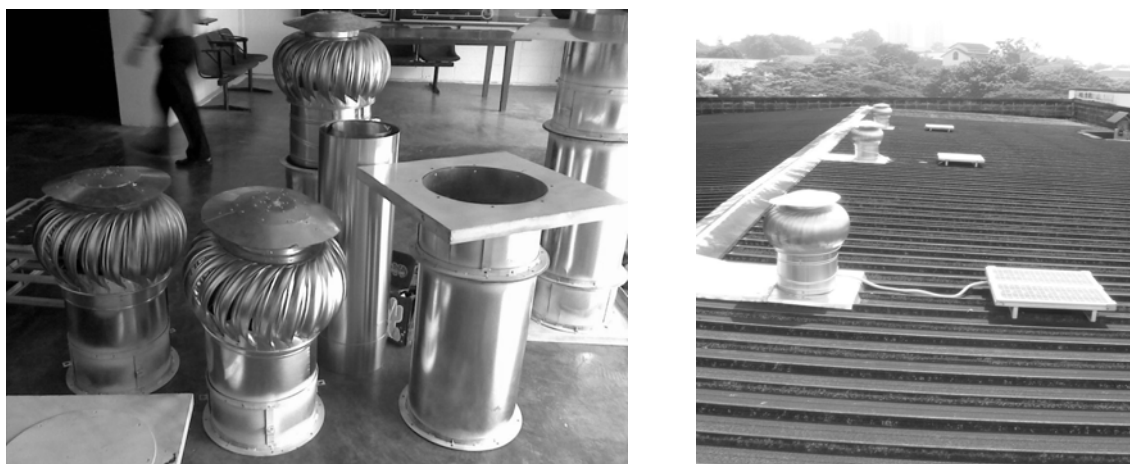
Fig. 2. Configuration of the HTV (a) before installation (b) three complete sets of the HTV installed on the roof
