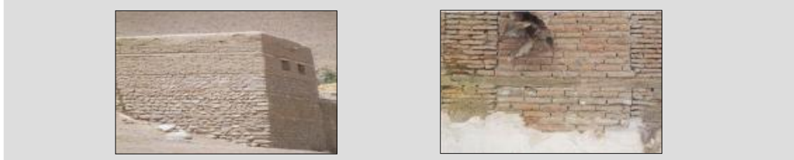
Figure 3- Picture on the right: The use of horizontal logs for strengthening walls with construction materials is a solution for increasing the building stability and resistance. Picture on the left: A rural house made of stone pieces with suitable joints at the corners with the rest of the stones lying in an oblique and regular manner (wedged left and right) with each row on top of the other
