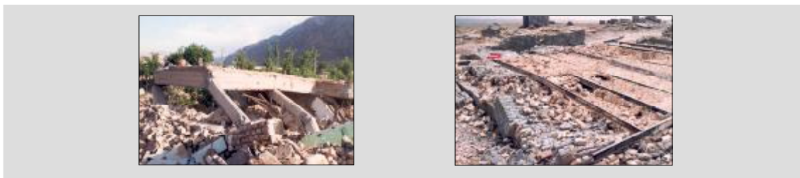
Figure 2- The heavy concrete ceilings and iron beams not connected at he vaulted ceilings are among the most important defects of new construction methods.
