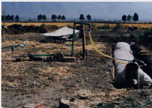
Figure 2. Installed polyethylene biogas plant.
