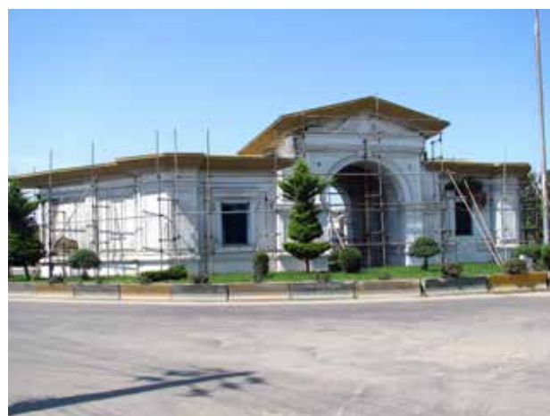
Fig. 10. The garden gate on northeast side, built during the reign of Reza Shah. Photo: author, 2010.
