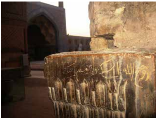
Fig. 3. Defacing, stone veneer, Eastern Eivan of Shah Mosque, in Naqsh-e Jahan Square, Isfahan. Source: www.sahebnews.ir
