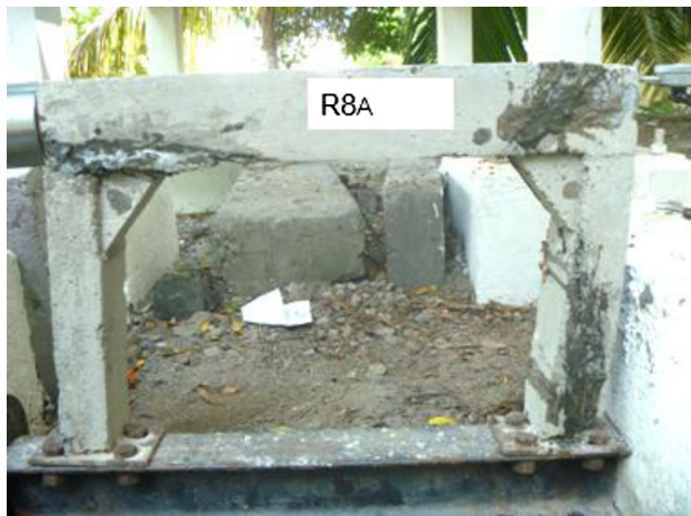
Fig. 8 Epoxy repaired, with partial concrete infill corner braced frame
