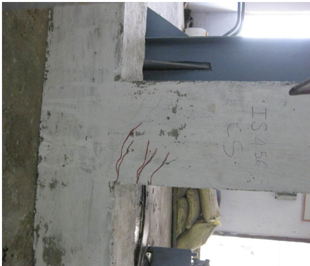
Fig. 9 Crack pattern of IS 456 CS
