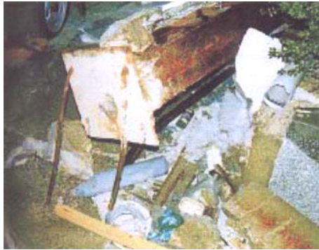
Fig. 2 Exposed column base pullout failure, Kobe (1995), Hitaka et al. (2003)
