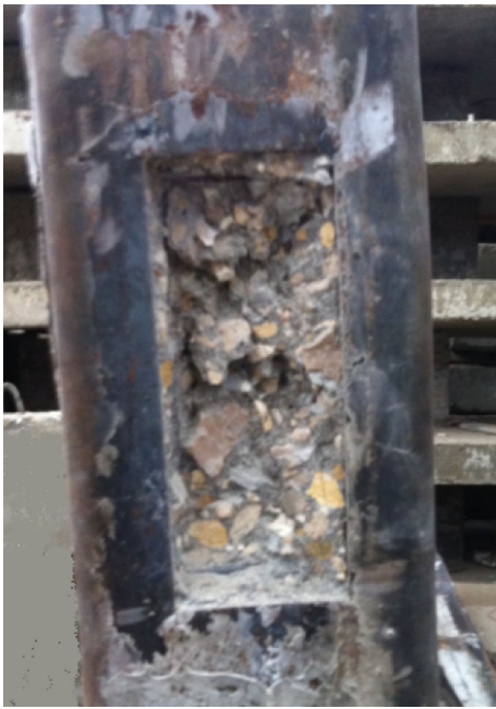
Fig. 11 Typical mode of failure for strengthened RC column using steel angles and strips
