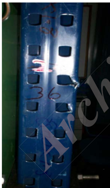
Fig. 8 Damage of the upright
