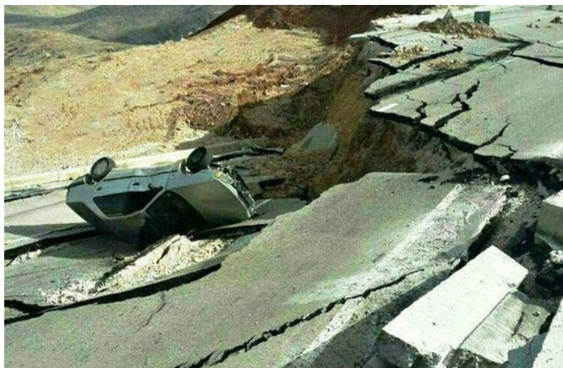
Figure 1: Land subsidence in a road, Fars province, southern Iran
