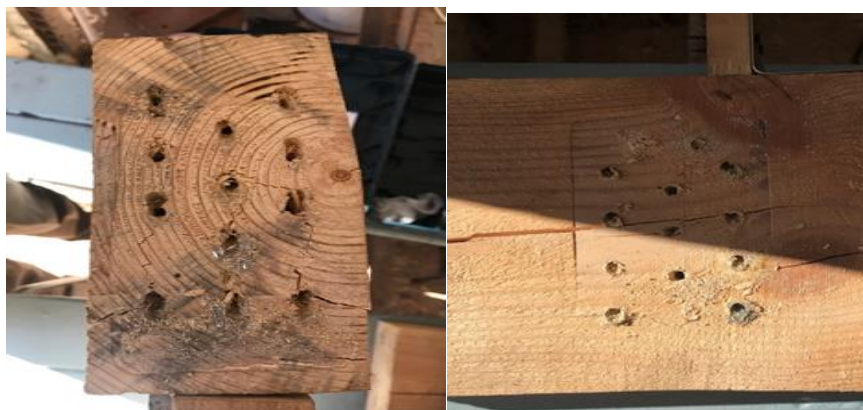
FIGURE 9 The nature of beam joint destruction:( a) secondary beam and (b) main beam
