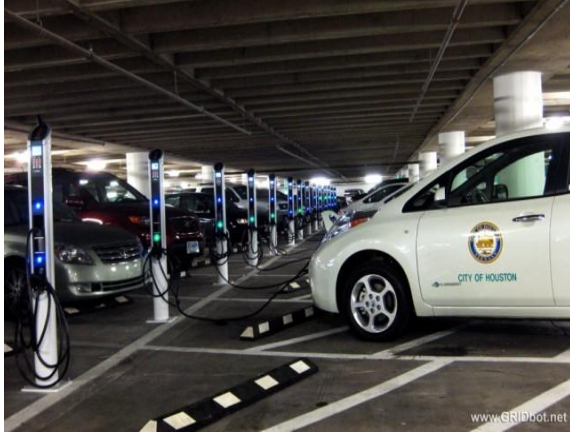
Fig.1. A parking lot supplying electric vehicle
