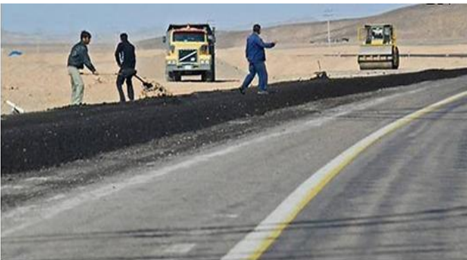
Fig.6. Road construction has affected natural habitat of A. farsicus in Maharlu basin.
