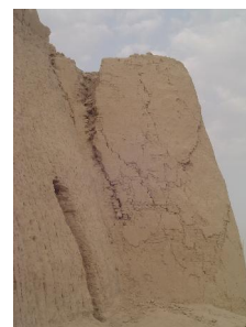
Fig. 6. Detachment between two walls in a corner
