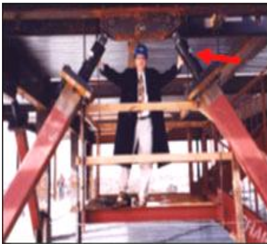
Fig. 5. Passive Energy Dissipation includes the introduction of devices such as dampers to dissipate earthquake energy producing friction or deformation [7]
