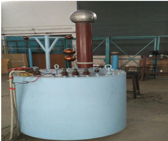
Figure 2. Transformer of 391V/150 KV, I-phase 30 KVA
