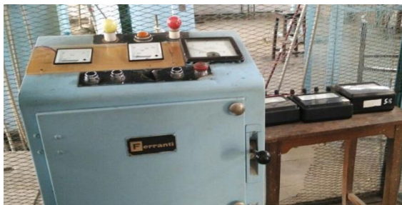
Figure 3. Voltage regulator at primary side of transformer
