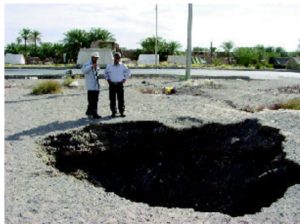
Figure 17. Large sinkhole observed at west of Baravat.
