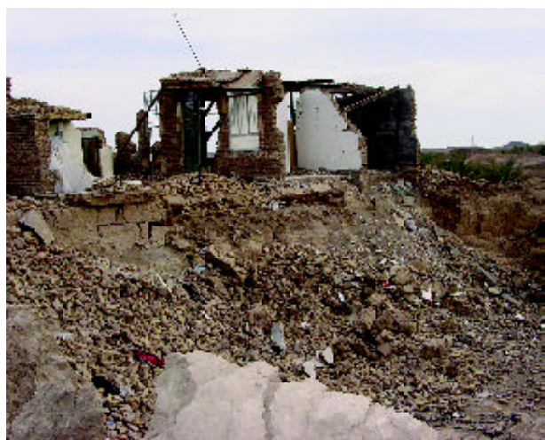
Figure 30. Damages to a building located at top of an excavation due to landslide, Esfikan village, Northeast of Bam.
